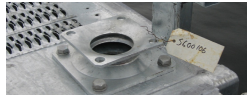
Lamp post connection point
